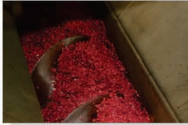
Seed Waste Conveyor
